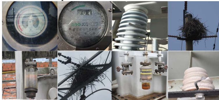
Fig.4 The Dataset Obtained from Substation.
